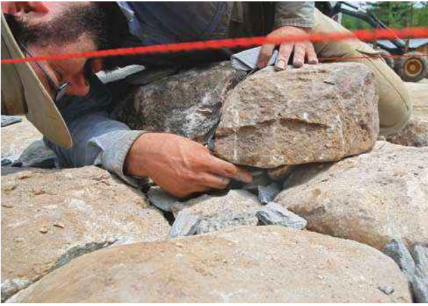
Pin from within. Pinning stones shim the face stones level and solidify their placement. Never pin from the face of the wall because it will just fall out over time.
